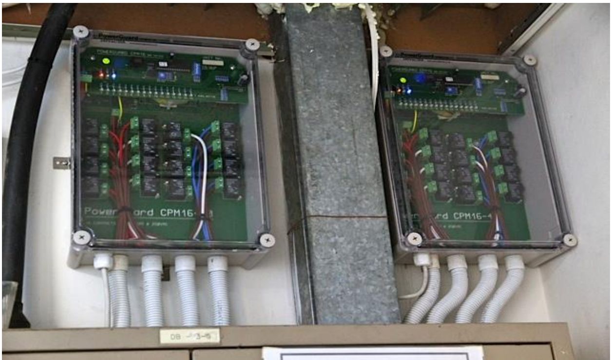
Figure 5: Two of the fourteen 16-channel controllers at defence contractor.
